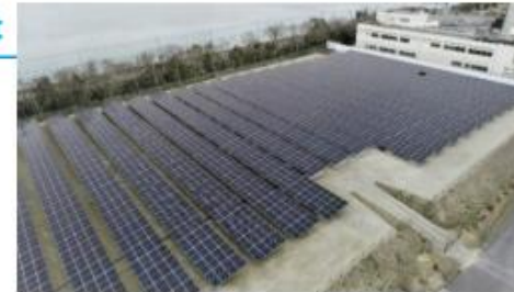
PPA model Large-scale Solar Power Generation Facility
